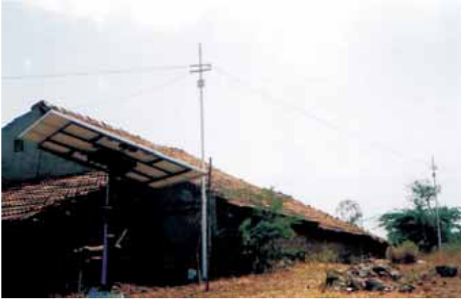
Figure 5 Pole-cable network in a cluster
